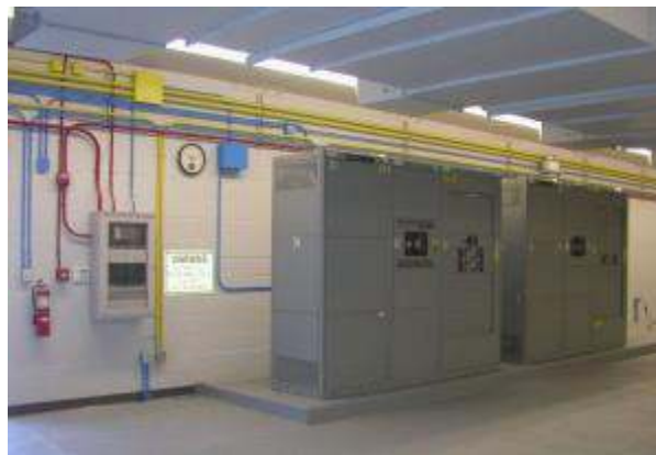
Gambar 2.19. Main Distribusi Panel
