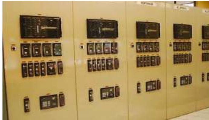
Gambar 15.12. Panel Proteksi (Protection Panel/ Relay Panel)
