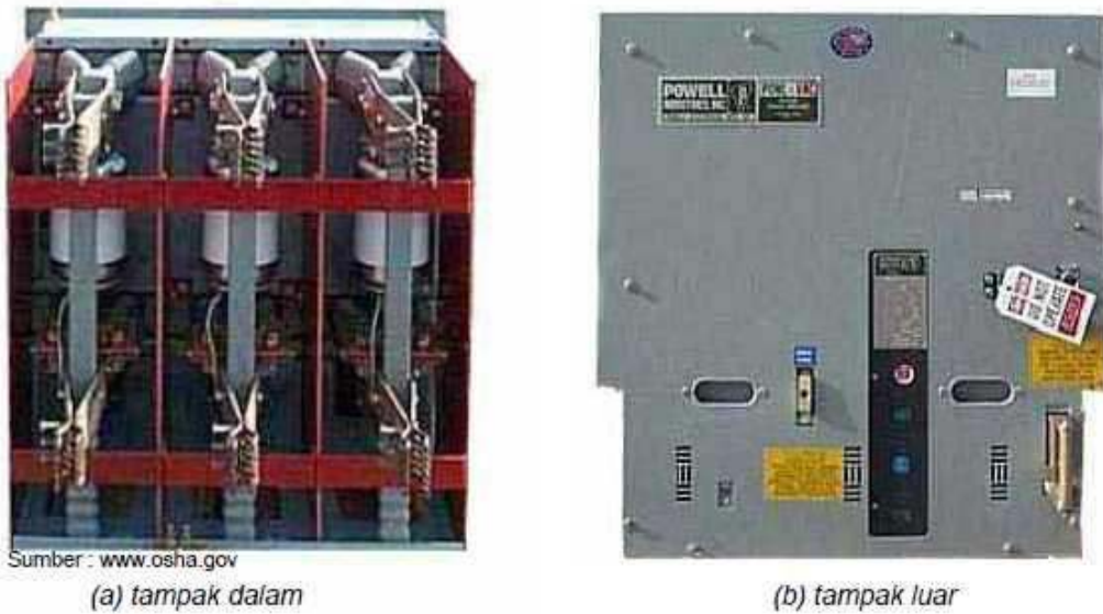
Gambar 1.46. VCB (Vacuum Circuit Breaker)
